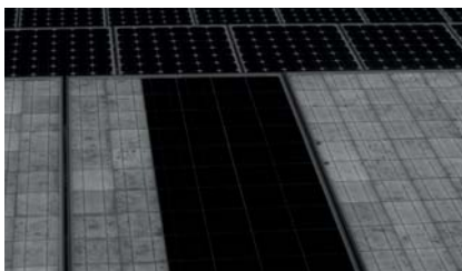
The electroluminescence image shows 2 defective bypass diodes
