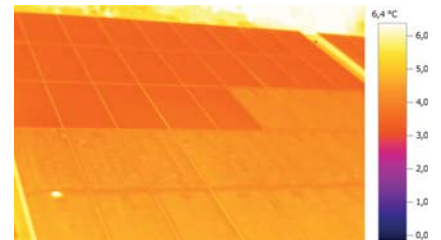
Solar module with a hotspot on the junction box
